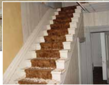
Central stairs with the bannister vandalized.
